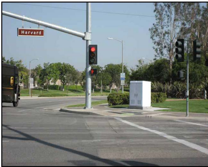
Figure 6: Traffic Signal Control Box 14
