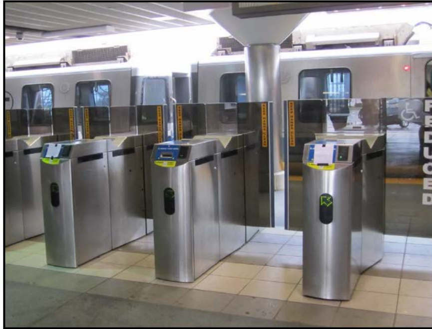
Figure 15: Passenger Access Control Gates at a Subway 26
