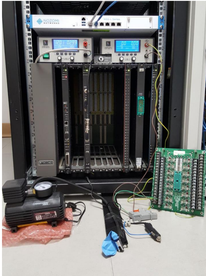
Figure 3 – Working Triconex infrastructure used to demonstrate successful TRITON OT infection
